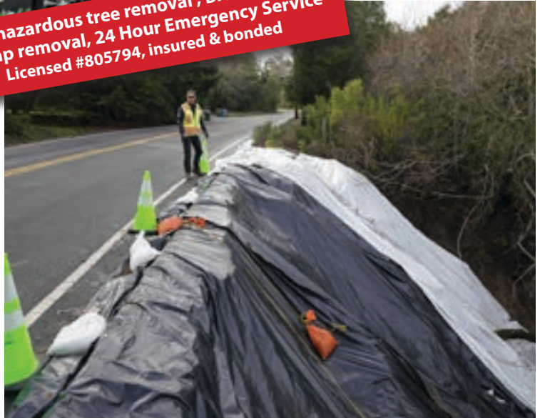
Public Works Director Mike Moran inspects segment of storm damaged shoulder of St Mary's Road near Driftwood Drive
